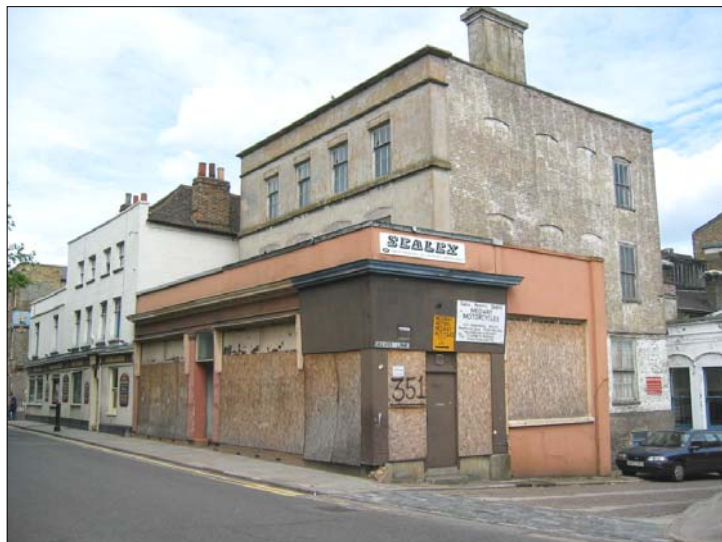
351 High St, building on the at risk register
