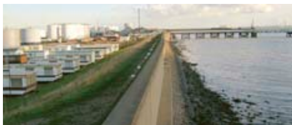
Flood defences at Canvey Island
